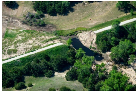
Figure 2. The Cowboy Trail runs 195 miles across northern Nebraska, following the old Chicago & Northwestern rail route from Norfolk in the east to Valentine in the west. In 2019, the trail flooded, causing serious damage, including one 100-foot-long section washed out by water. Image source: Outdoor Nebraska Magazine
